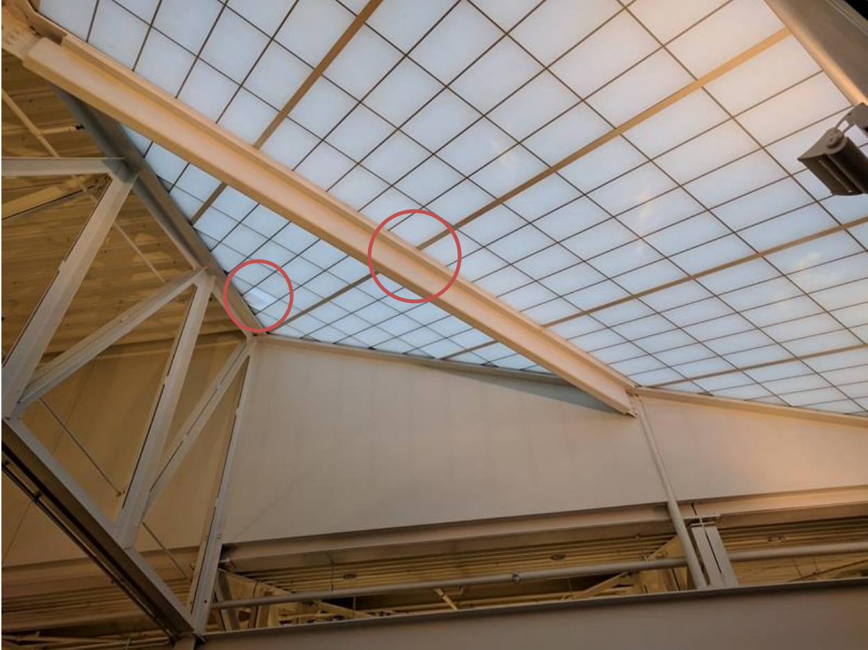
Leak location as well as panel insert issue
